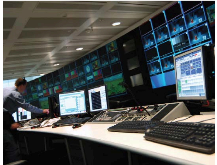
Commander digital matrix intercom installed at BBC London
